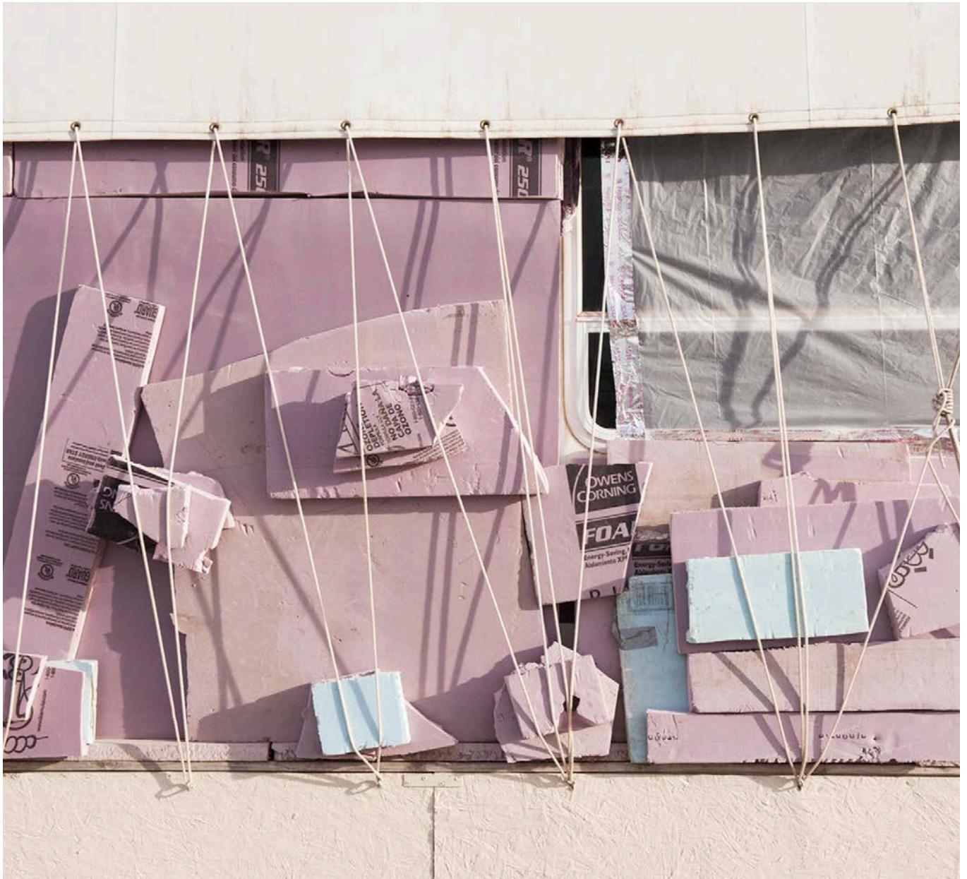
xvii Photo taken on site at an RV Camp outside of Williston / Makeshift thermal additions for use during winter months.
